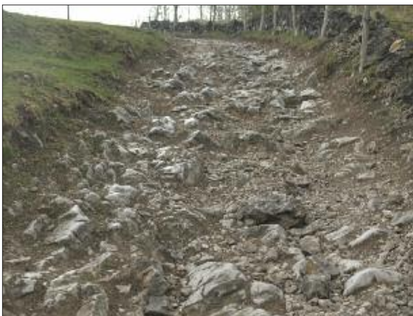
This part of Brushfield used to have a good surface. Horse riders could canter up it. It is now impossible on horseback.
